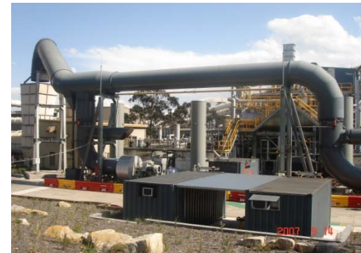
BHP Billiton Illawara Coal , West Cliff Colliery, Australia, 150,000 CFM, 0.9% CH 4 , 6 MW Power
